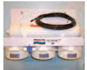
RO Unit mounted on wall
