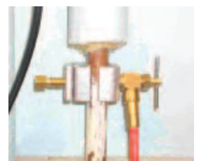
Supply Pipe Saddle CLOSED
