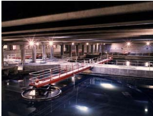
Settling Tanks at the Winnipeg Wastewater Treatment Plant
