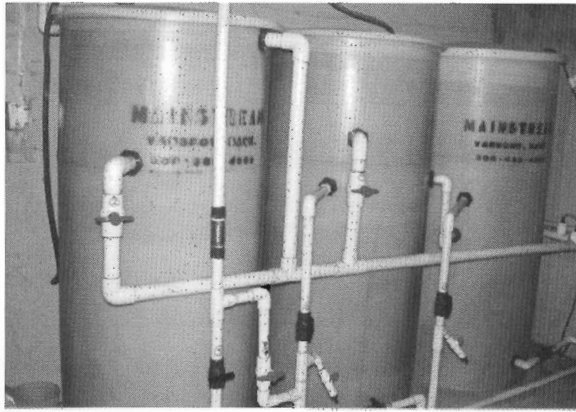
Fig. 2. An experimental groundwater treatment system manufactured by Mainstream BMS Ltd.
