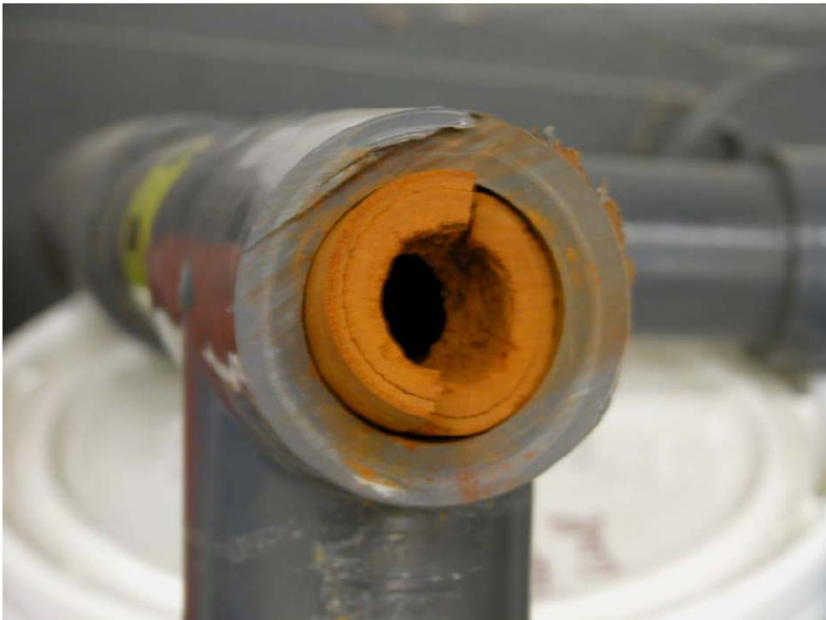
Picture1: A thick layer of iron bacteria growing inside a water pipe
