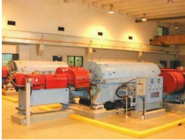
Centrifuge at the Winnipeg Wastewater Treatment Plant
